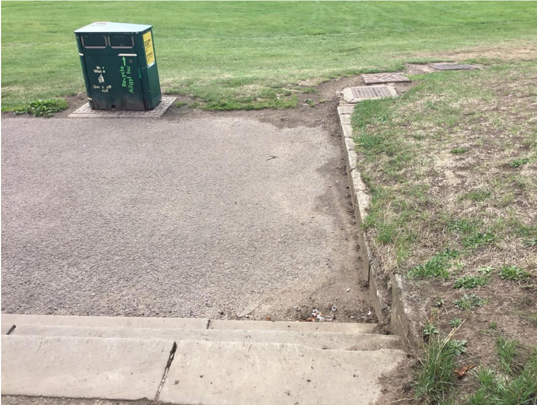
Same access path - steps at bottom. Note: there is no provision of ramp or alternative access to the land for wheelchair users and anyone with mobility problems. Those with prams/buggies may also struggle if they are alone
