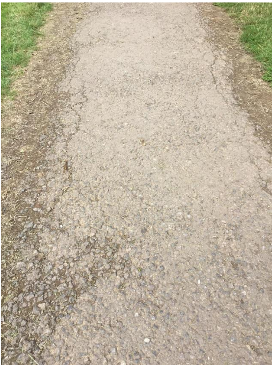
Path from car park has been allowed to deteriorate considerably and likely to be an obstacle for wheelchair users to access the land "of equivalence"
