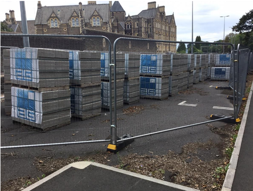
Nearest available car parking spaces suspended for considerable period of time while substantial works are undertaken
